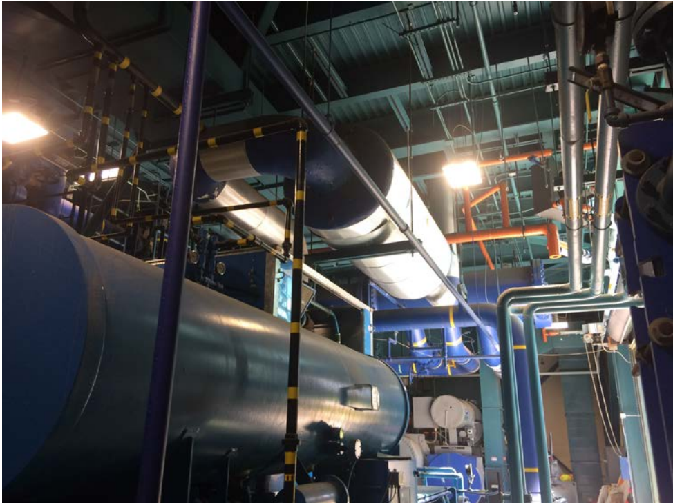
Existing Chiller 3 to be replaced at left
