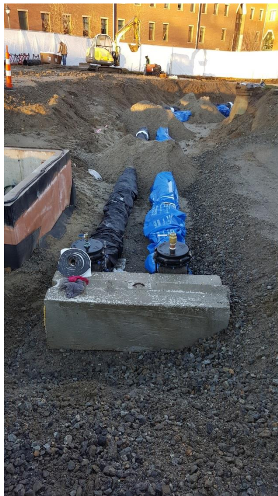
Installation of domestic water and fire main connections to existing utility tunnel
