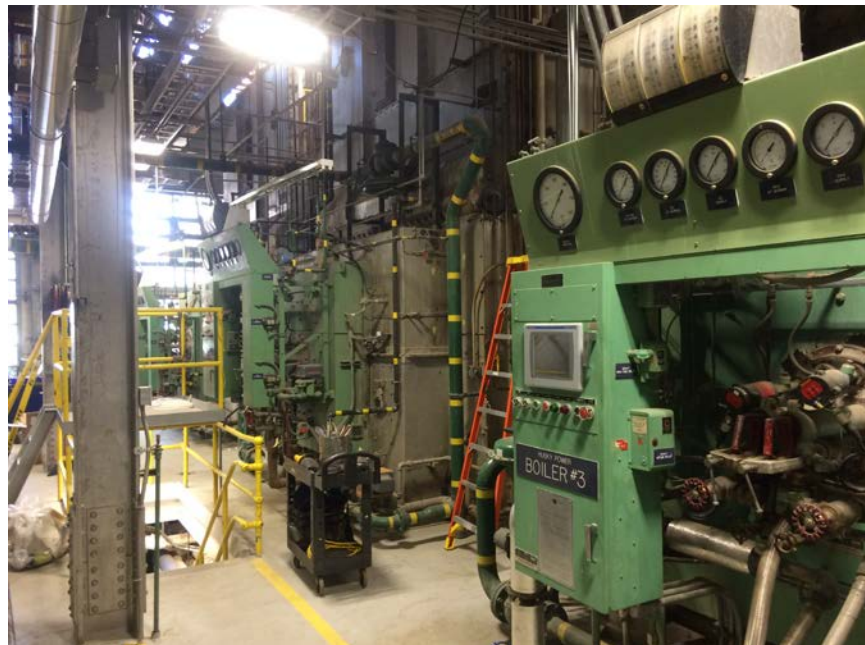
Existing CUP Steam Boiler 1 (1960), Boiler 2 (1962) and Boiler 3 (1966)
