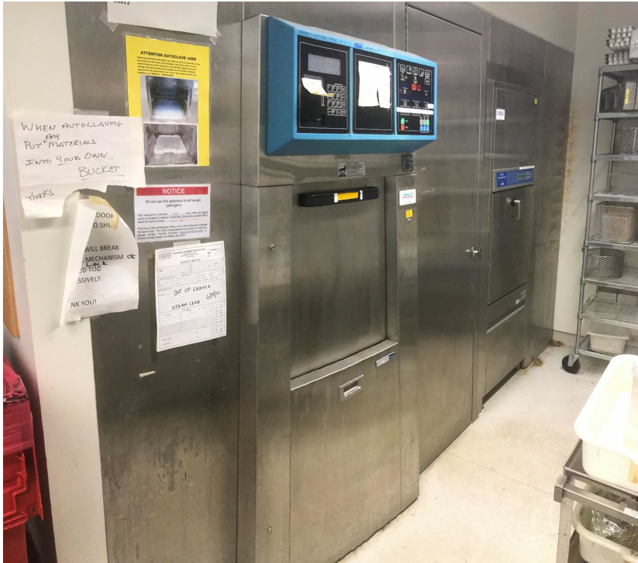
Broken Autoclave and Washer in the Academic Research Building
