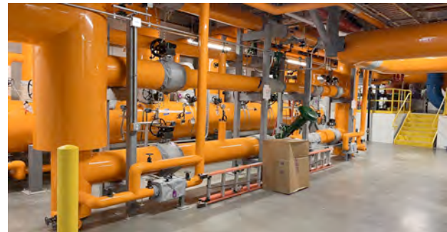
SUP Interior View of 125 psi Steam Header
