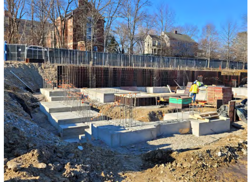
Foundations Installed at a portion of the new Residence Hall near Academic Way
