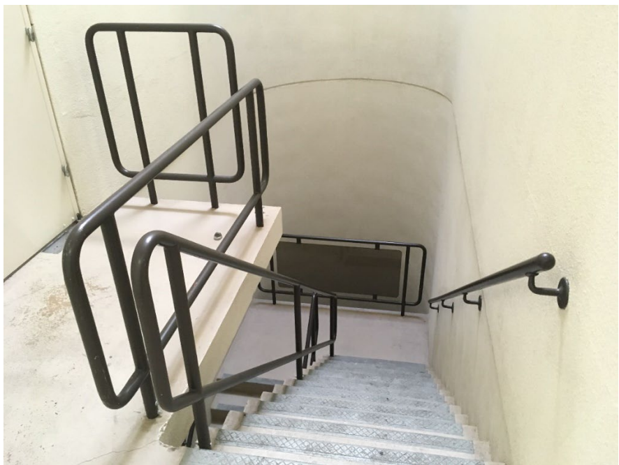
16 MUNSON ROAD NON-COMPLIANT EGRESS STAIR RAILING
