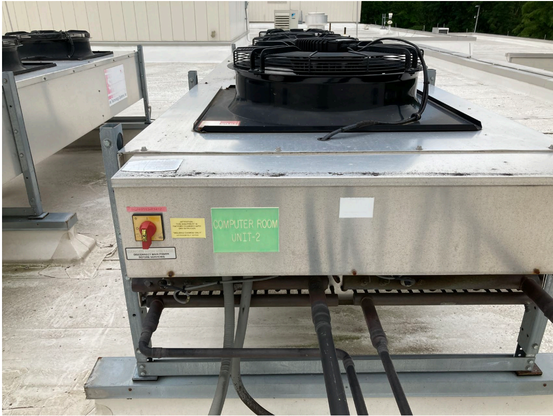
ROOF TOP COOLING UNIT
