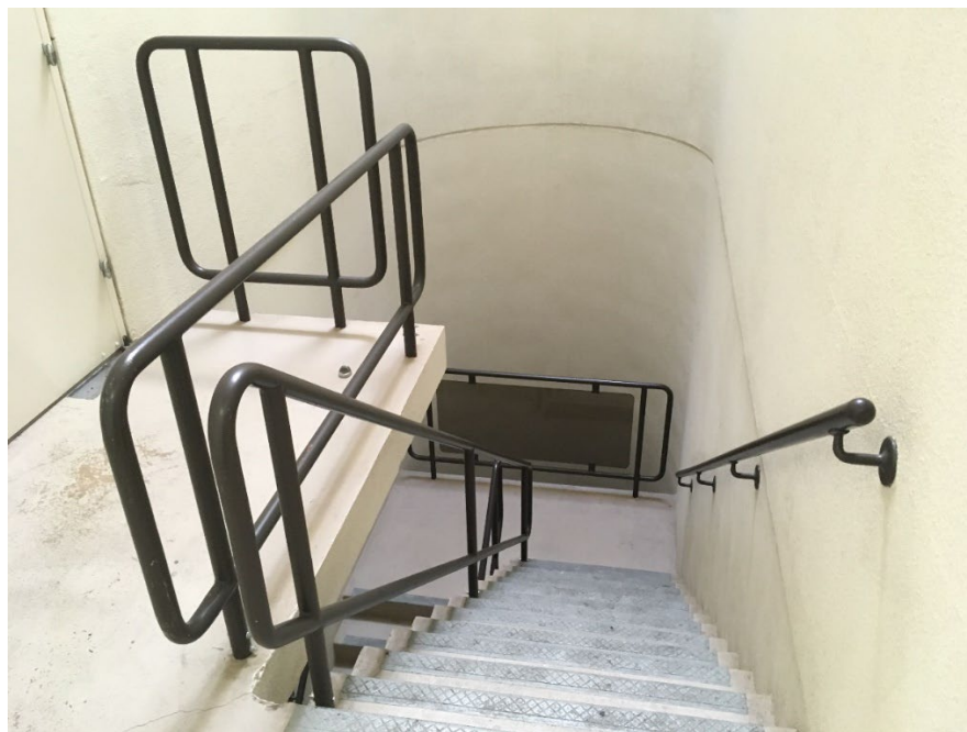
16 MUNSON ROAD NON-COMPLIANT EGRESS STAIR RAILING
