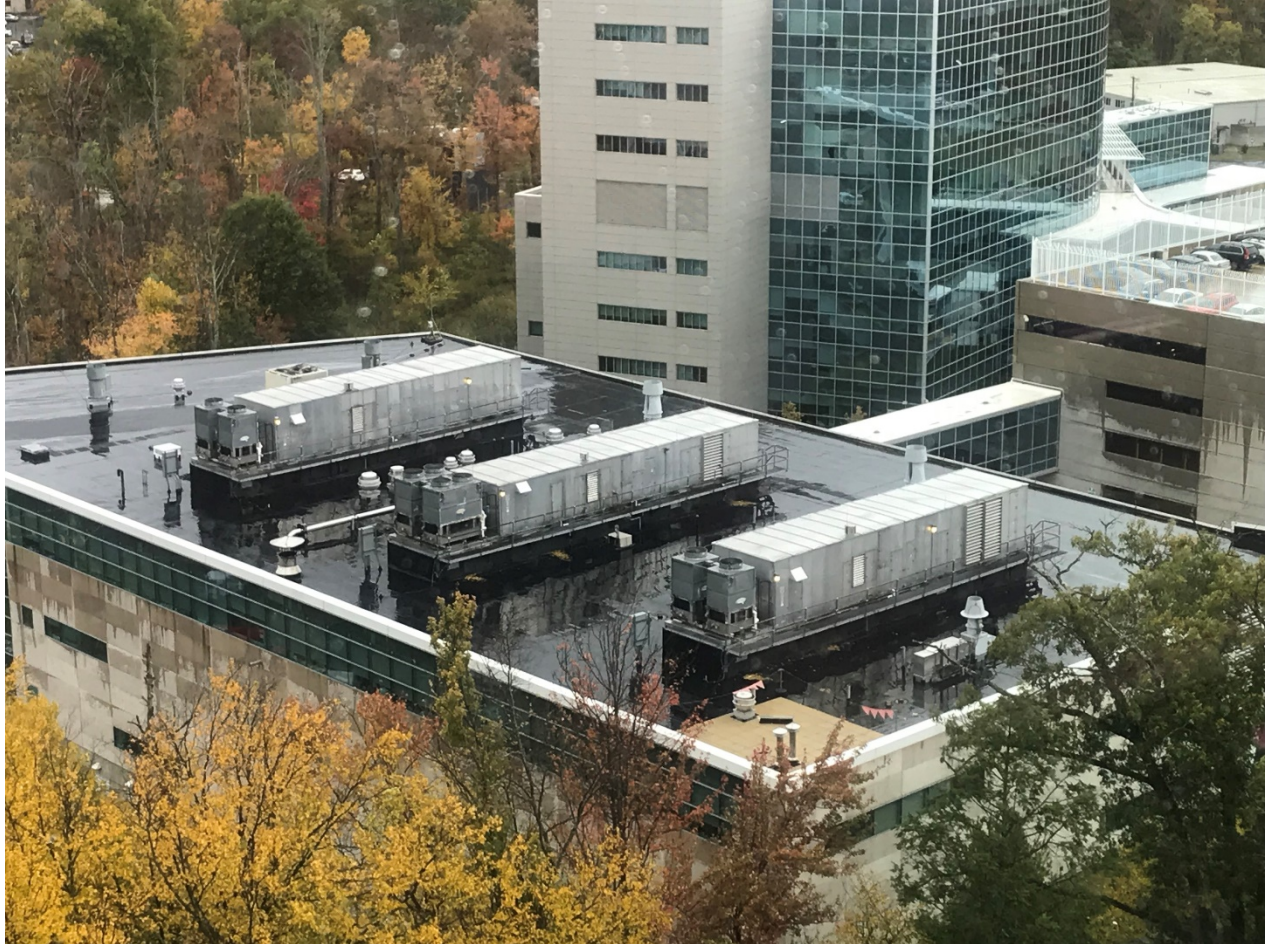
VIEW OF MSI BUILDING ROOF TOP UNITS #1, #2 & #3
