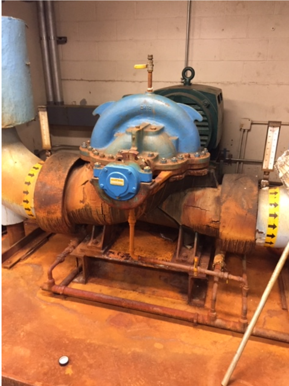
EXISTING CHILLED WATER PUMP #4
