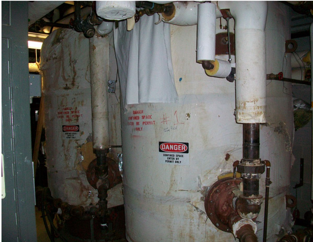
EXISTING STEAM-TO-HOT WATER HEAT EXCHANGER AND STORAGE TANKS
