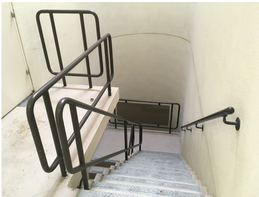
16 MUNSON ROAD NON-COMPLIANT EGRESS STAIR RAILING
